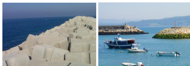
Figure 1. Picture of the antifers breakwater in Molfetta (Italy) and rubble mound breakwater in Muxia (Spain).
