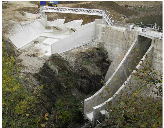
Figure 1. The Goulours dam spillways. The old ski-jump-type spillway is on the right, whereas the new PK weir appears on the left (under construction).
